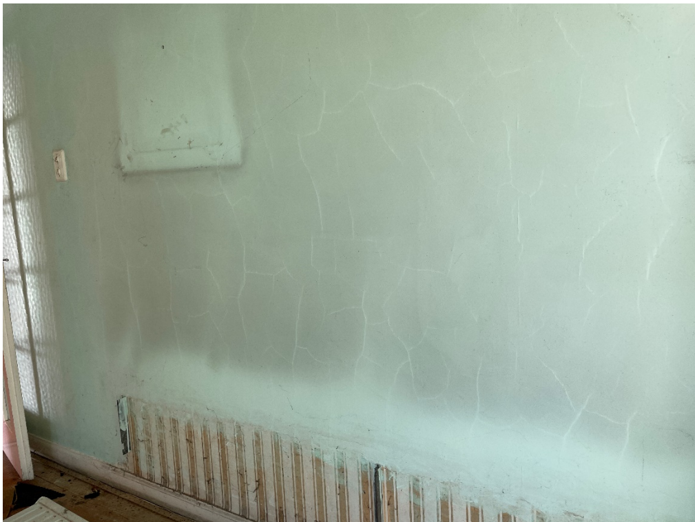
Photograph 12 – Cracking to internal face of external walls
