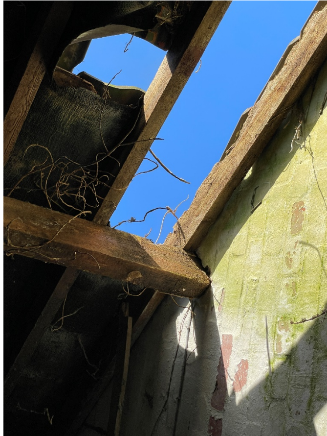
Photograph 5 – Poor roof condition in outbuildings
