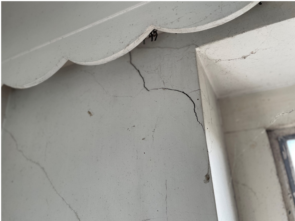
Photograph 10 – Diagonal cracking over doorway
