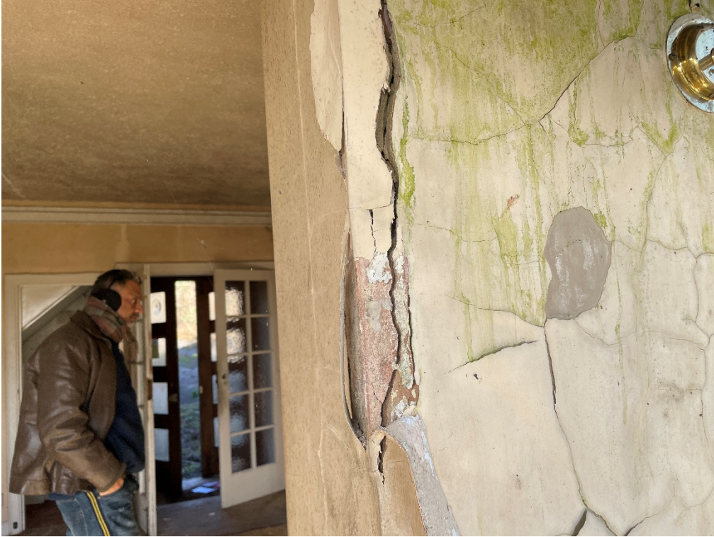
Photograph 7 – Vertical cracking into rear sun room
