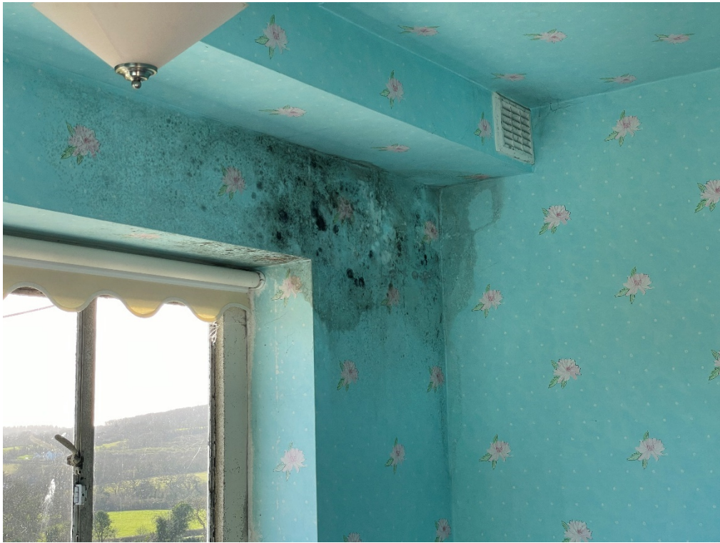
Photograph 13 – Damp areas throughout the property
