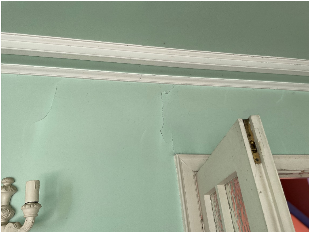
Photograph 11 – Vertical cracking over ground floor doorway
