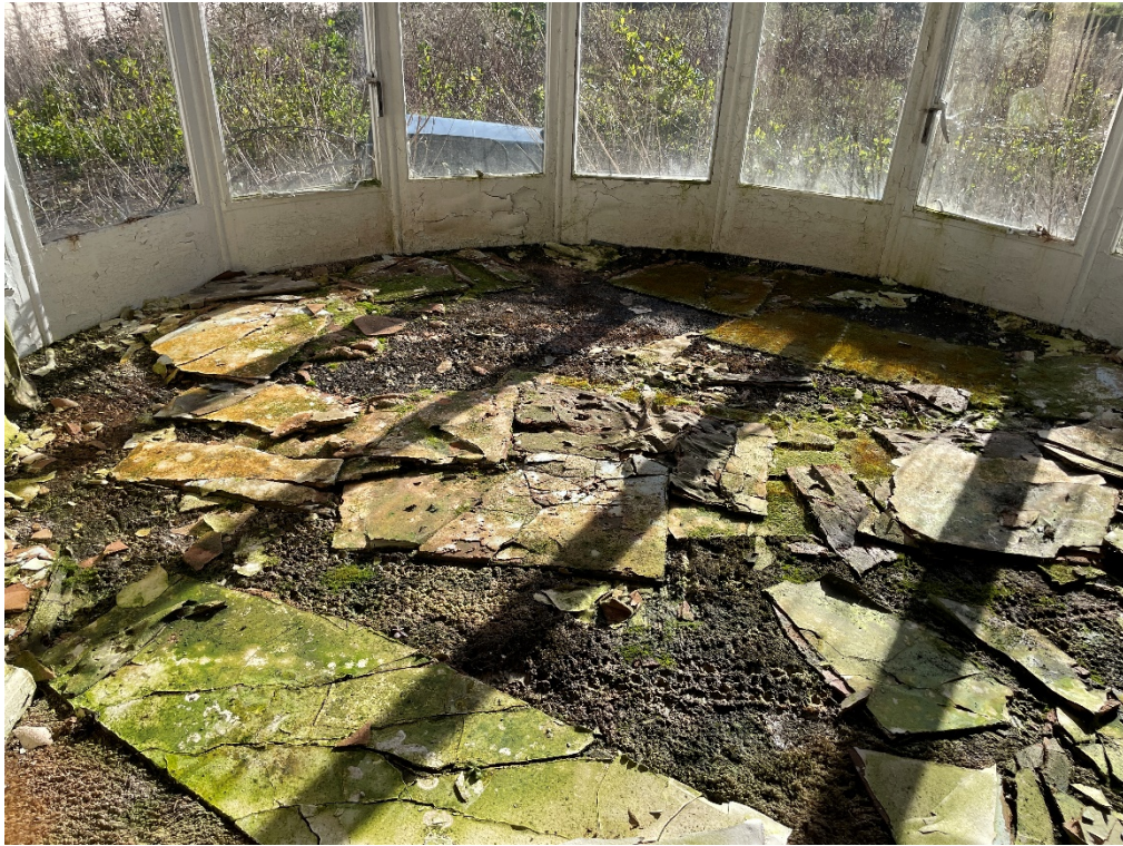
Photograph 3 – Poor condition of rear sun room
